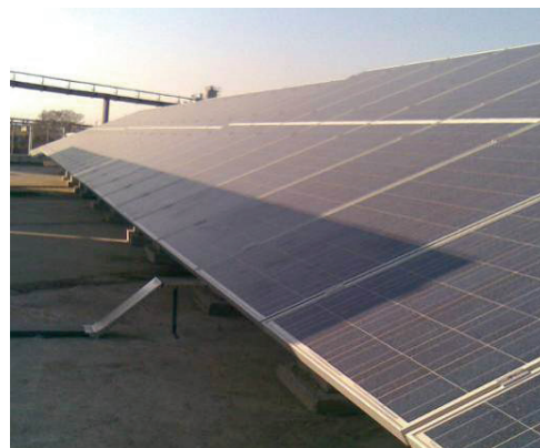
Figure 2: Grid-connected PV installation with a supporting structure that cast a shadow over the panels behind it.
