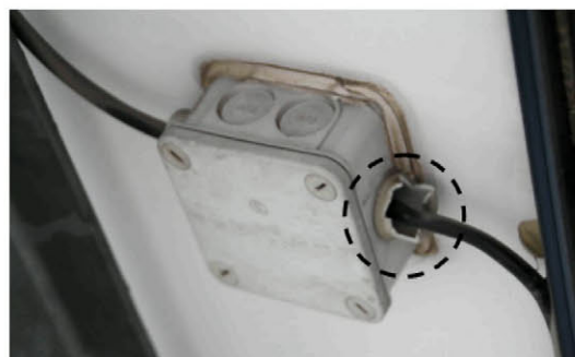
Figure 2. Cracks in the terminal boxes appeared during the first 13 years of operation.
