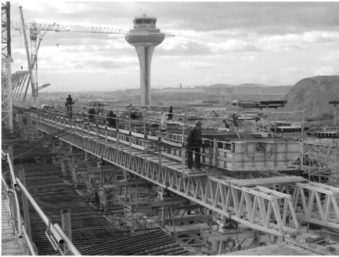
Fig. 1. Satellite Building T4 of the New Airport Terminal Barajas during construction (photograph by Tobias Petschke)
