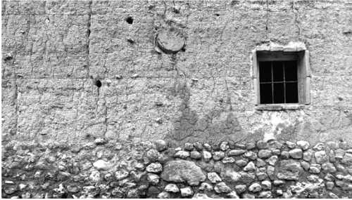
Figure 4. Rammed-earth wall in Almántiga. The window hole is made with bricks as formwork. (Credits: Gil Crespo).
