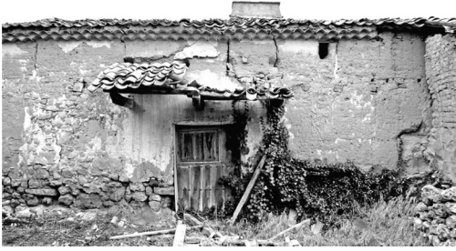
Figure 3. Rammed-earth wall in Covarrubias, with plinth of stone and parts with adobe. (Credits: Gil Crespo).
