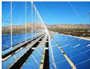
Figure 5: “Puerto Errado 1“ Solar thermal powerplant in Murcia, Spain
