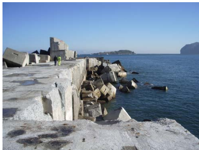
Figure 3. Port of Bermeo, Biscay (northern Spain). Slide failure and overturning in 2010
