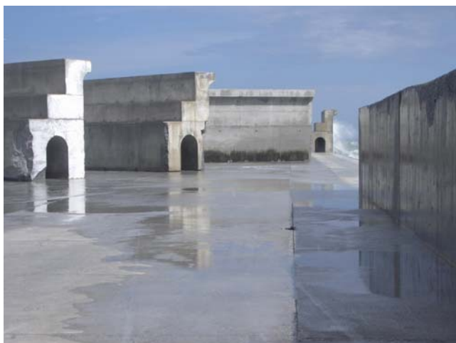
Figure 2. Port of Motril, Granada (southern Spain). Slide failure in 2004
