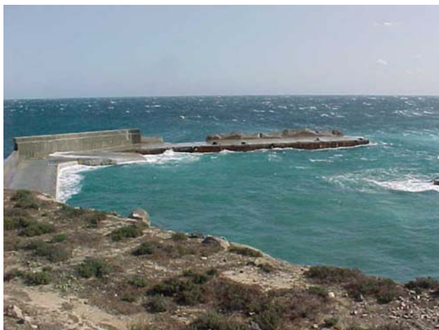
Figure 1. Port of the island of Alborán (southern Spain). Hammer shock failure in 2001
