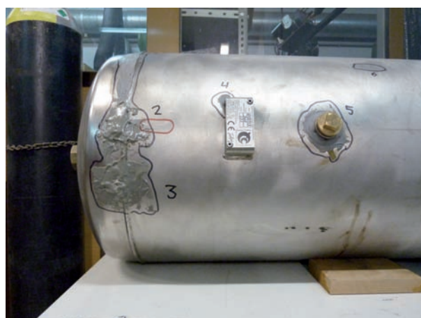
Figure 1. Aspect of the 250-L water tank around the lower zone (head 1). The repairs, made with resin, are seen.
