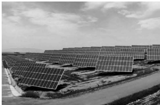
Figure 1. “Montes del Cierzo” PV plant.
