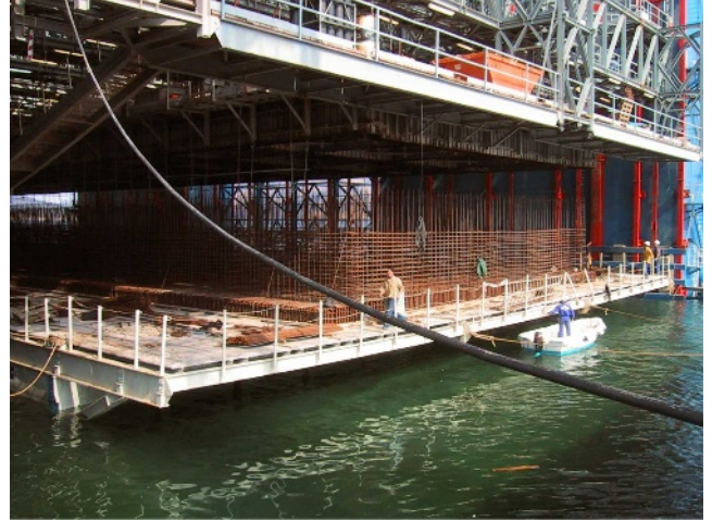
Figure 19. Close-up of the steel reinforcements being suspended in the floating dock umbrella
