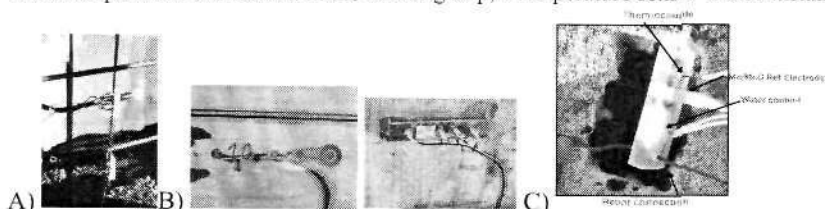
Fig. 1. A) Embedded sensors for electrochemical measurements installed in a dock in the south of Spain. B) Surface sensors installed inside a bridge. C) Passive sensors installed in Zarzuela Racecourse.
