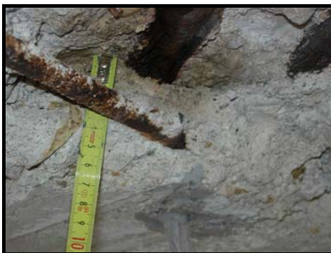
Figure 2. Measurement of the carbonation front in the shell.
