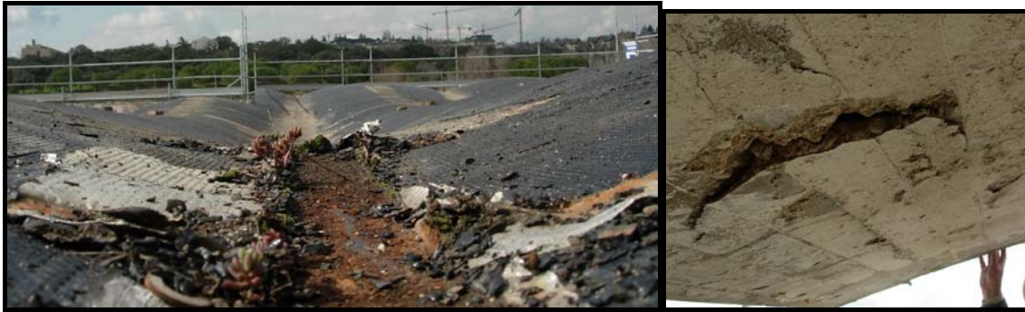
Figure 3. Deterioration observed before the restoration: Left: Lower part of one deck. Right: loss of upper waterproofing foil
