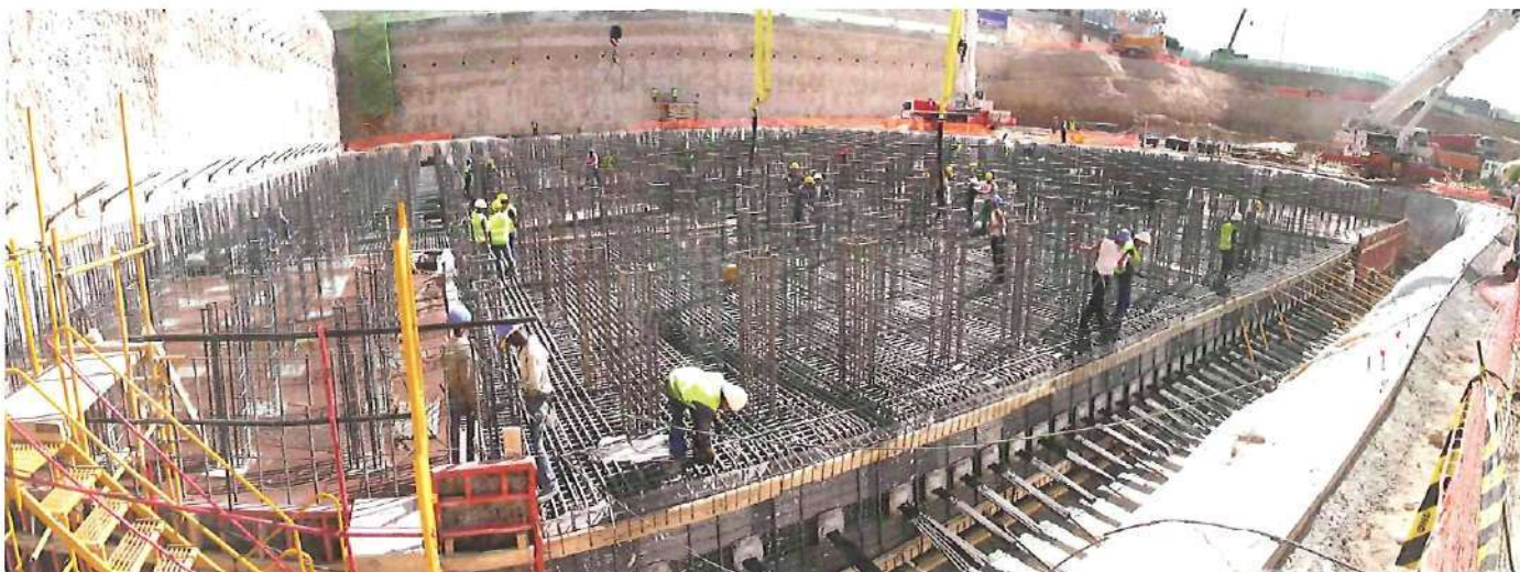
△ Figure 2 General view of the foundation mat at Torre Espacio including the prestressing cables
