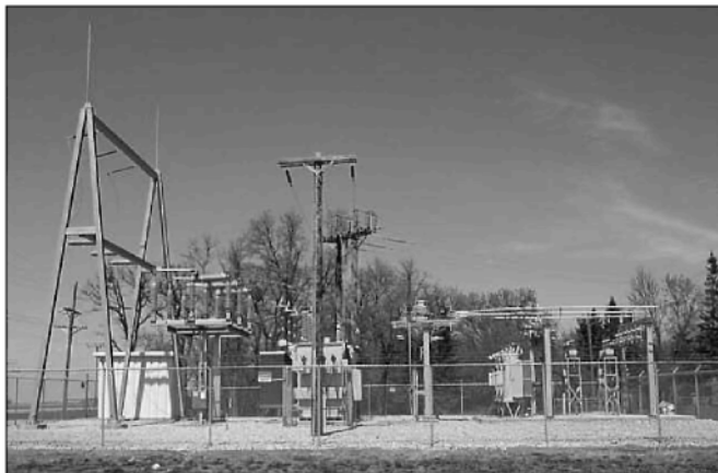
Figure 1. Real electrical substation
