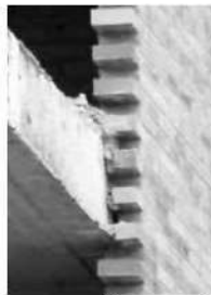
Figure.1. Traditional Spanish enclosure wall over-hanging on the edge of the floor slab.
