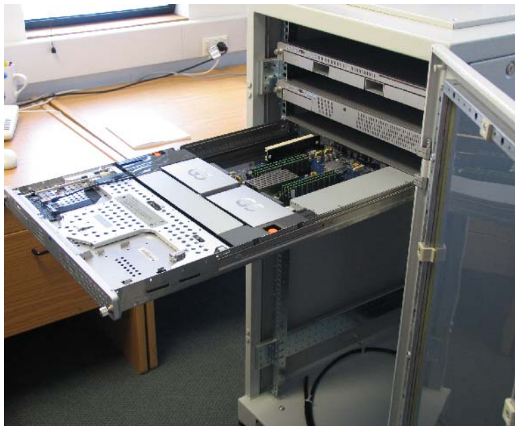
Figure 1: The 24-Unit Rack cabinet containing a partially constructed “Monte” dual-G5 compute cluster.
