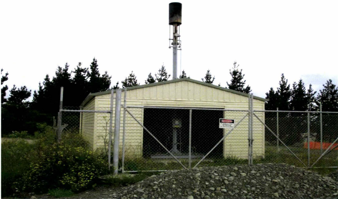
Figure 4.4. Gas flare station at Awapuni landfill
