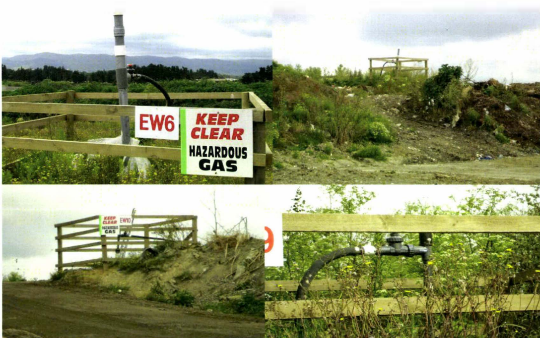
Figure 4.5: Methane collection system installed at Awapuni landfill
