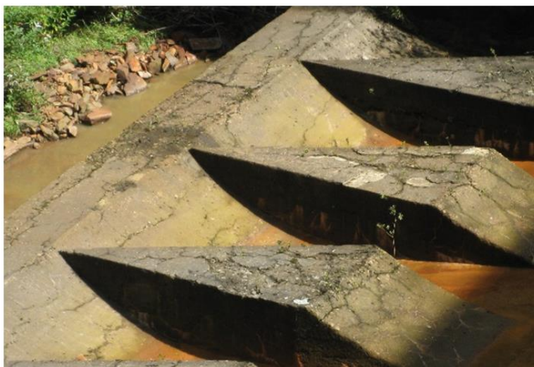
Fig. 6.- Cracks in an annexed structures
