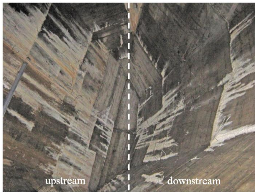
Fig. 13.- Calcium carbonate in joints
