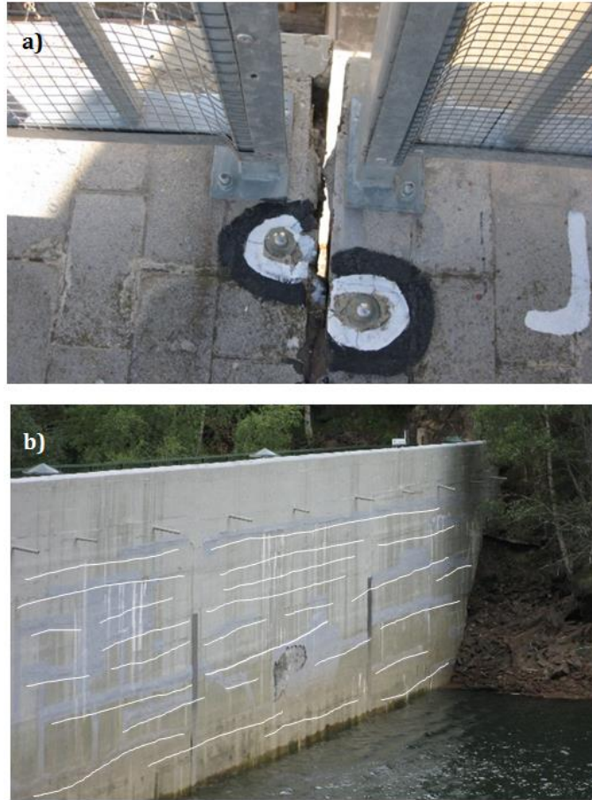
Fig. 5.- Damages in dams: a) remaining movements; b) Fissures upstream face
