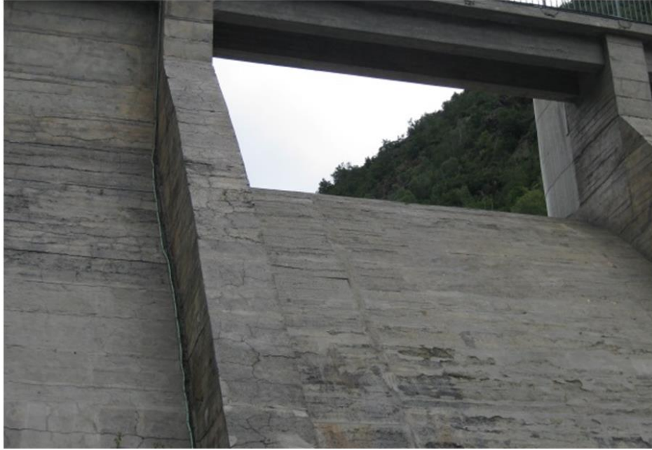
Fig. 7.- Damage in a dam: downstream face body and spillway
