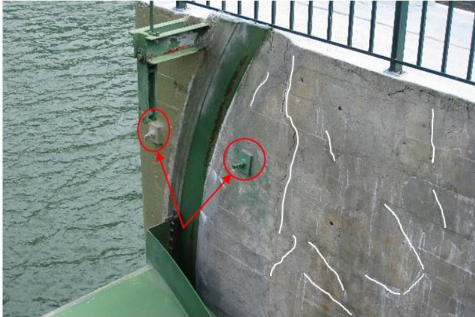
Fig. 9.- Gate area with cracks
