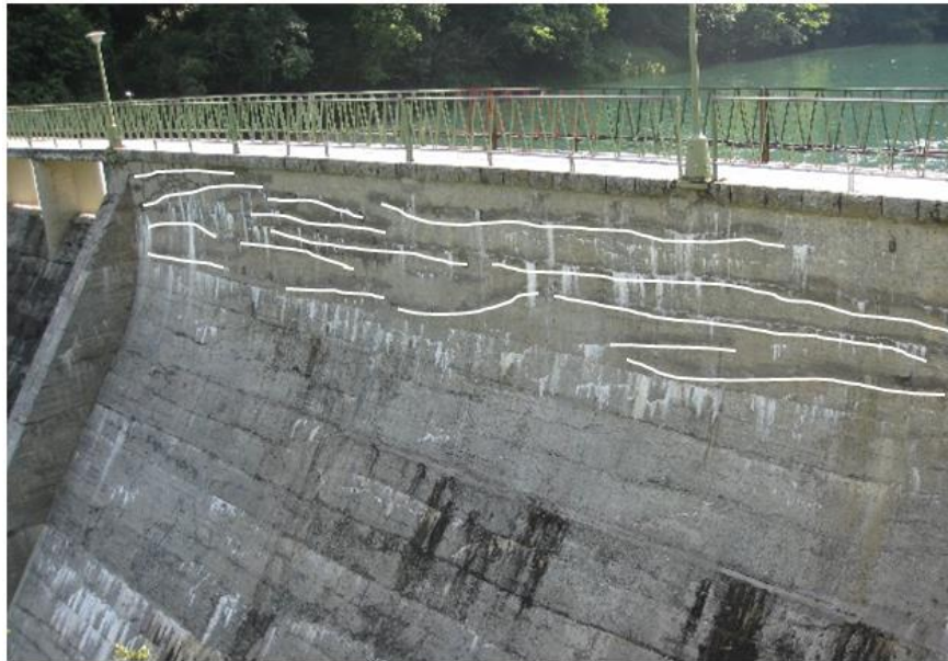
Fig. 4.- Horizontal fissure on a dam body
