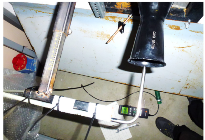
Fig. 5. Implement for measuring the air speed in the centre of the air spout.
