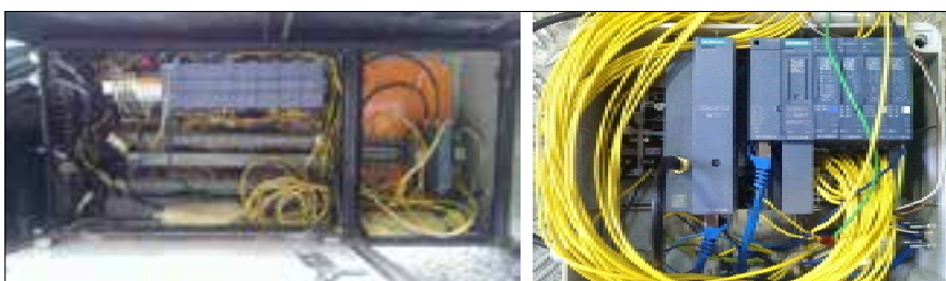
Figure 4. Main distribution cabinet after reconstruction procedure
