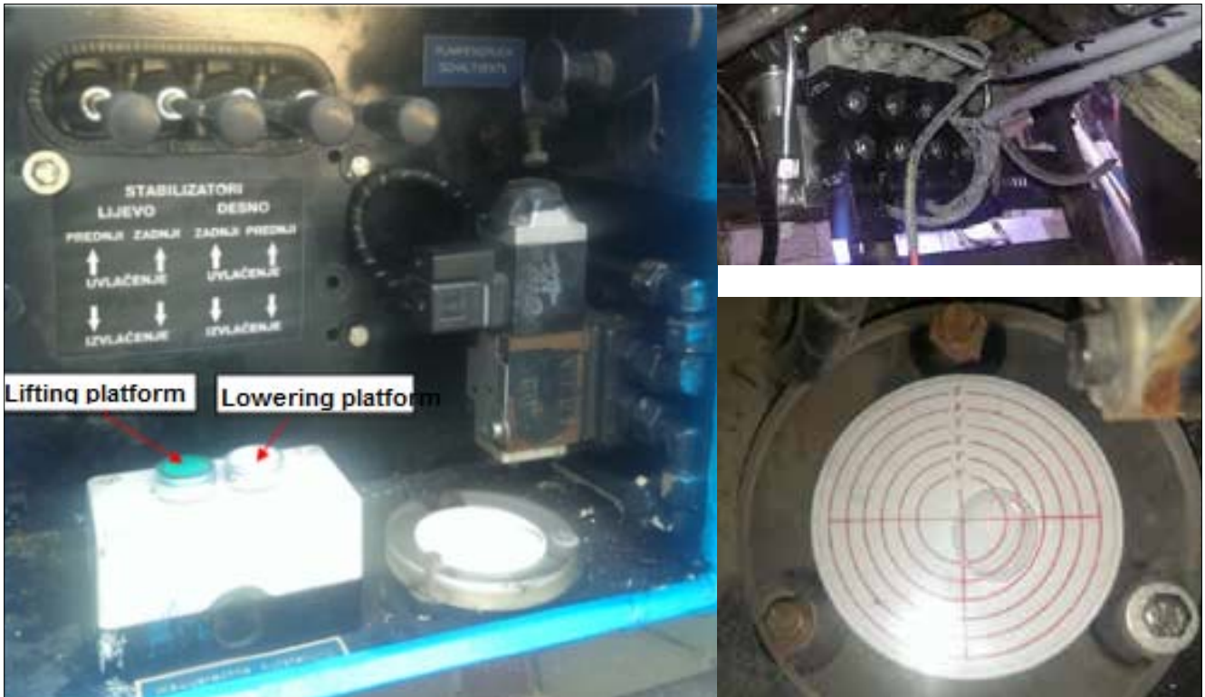
Figure 3. Cabinet for automatic levelling after reconstruction procedure, hydraulic distributors for nivelation process and circular libelle
