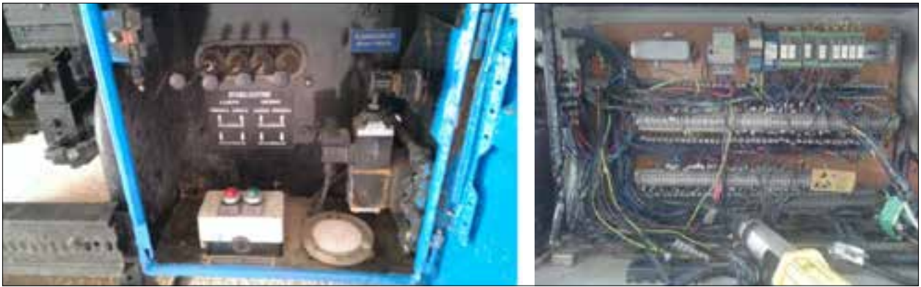
Figure 2. Cabinet for levelling process and main distribution cabinet before reconstruction
