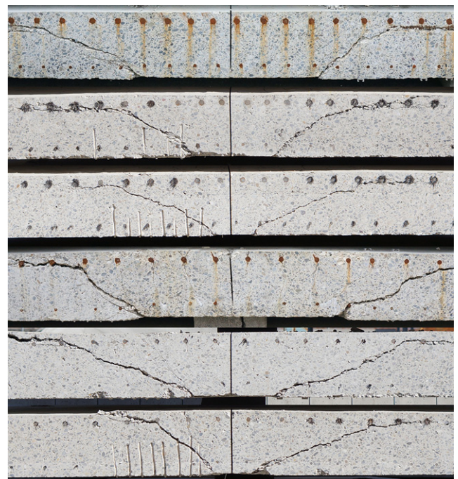
Figure 5. Photographs of saw-cuts of the specimens along the E–W axis (from top to bottom: PE5, PE8, PE7, PE12, PE9, PE11, i.e. decreasing column size and reinforcement ratio)
