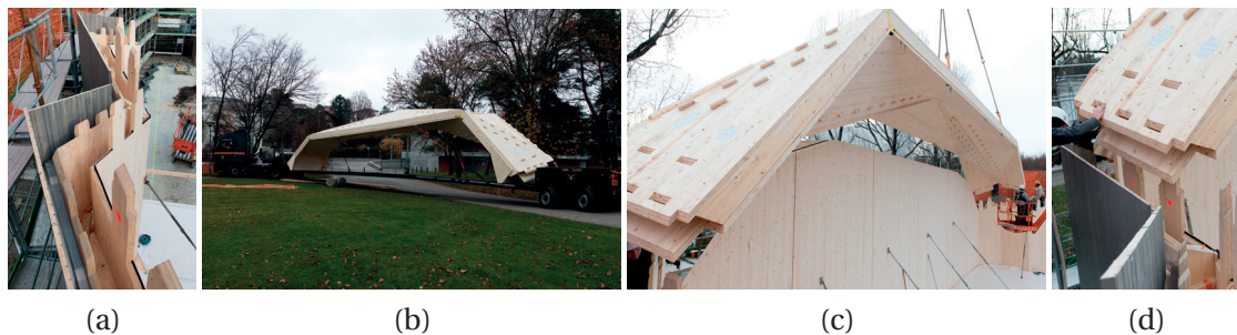
Figure 2.16 – Vidy theater erection [RGCW16] : (a) External wall with cladding, (b) pre-assembled roof element on a trailer, (c) Roof element lifting and (d) Insertion of wall tab into roof slots
