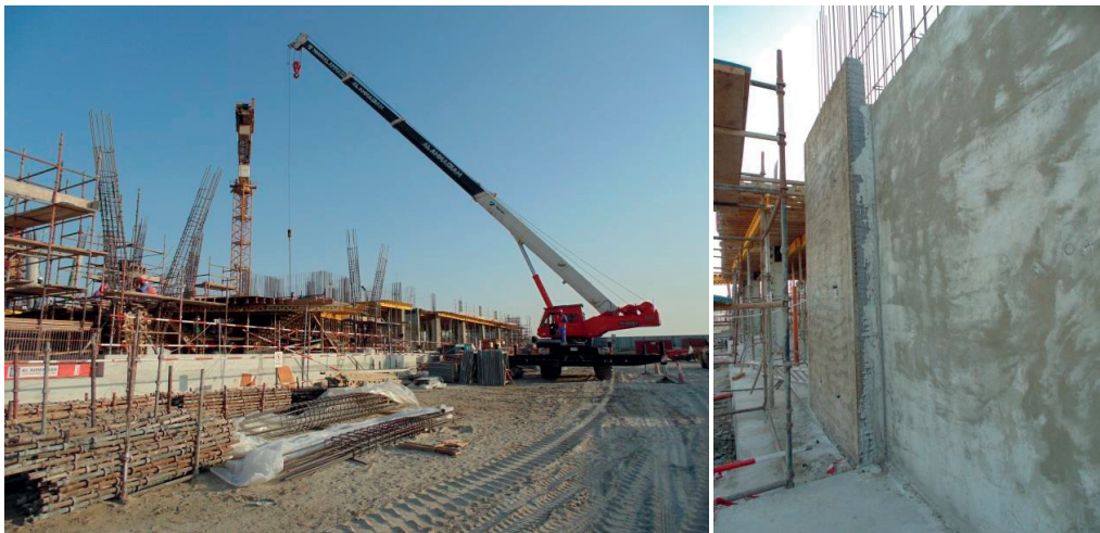
Figure B.5 Swiss International School Campus in Dubai. View of the construction site, 11 th November 2014. Main building (left) and detail of the walls (right).
