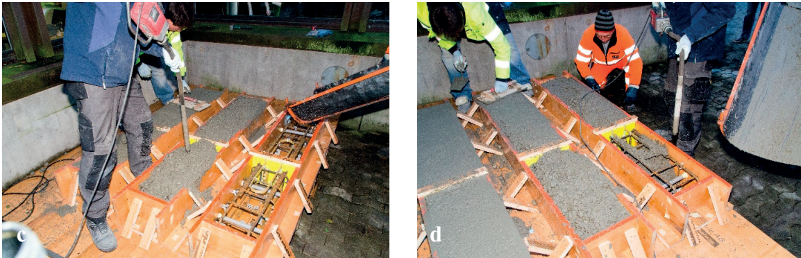
Figure G.1. Beam casting, 2 nd series, a) Formwork and steel reinforcement of beams, b) pouring of concrete, c) concrete vibration, d) smoothing concrete surface.
