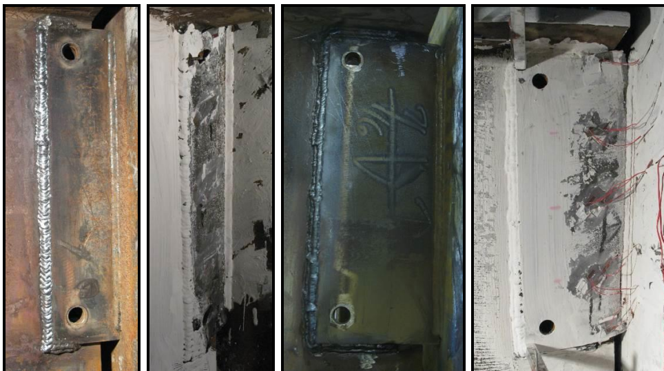
Figure 10: Photographs of post-test deformations for welded connections “Partial C” weld on replacement shear tab plate (Test Configurations 12 & 13)
