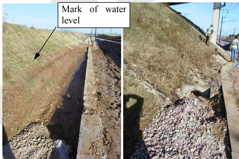
Figure 2: Damages observed aside the track 1 (on the left) and track 2 (on the right)
