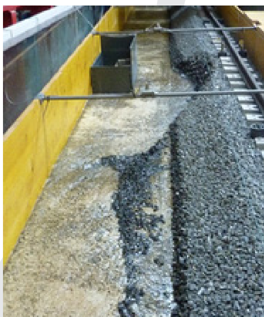
Figure 11: Impact on the ballast of runoff through the reduced section of a road bridge abutment
