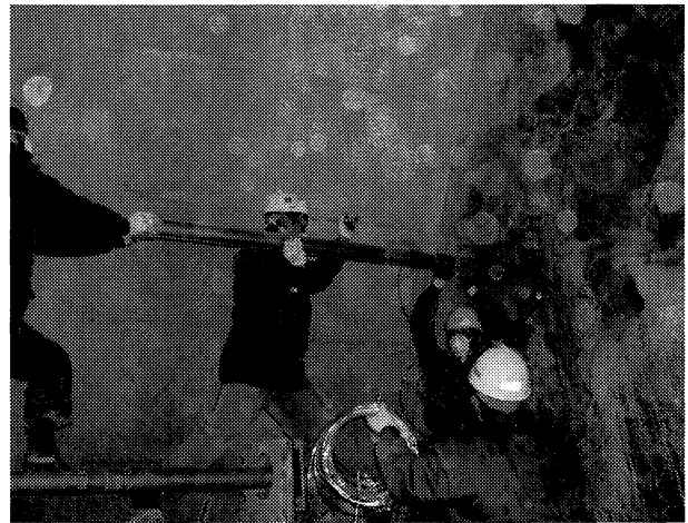
Fig 4 Installation of a reinforcing pipe containing fibres as strain sensor in the Ulsan-Kangdong tunnel.
