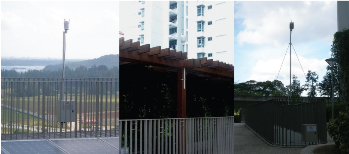
1 2 Figure 7: Installation of the weather stations (left: on roof; middle: on eco-deck trellis; right: on eco- 3 deck railing) (modified from Pan ShanShan 2 ).
