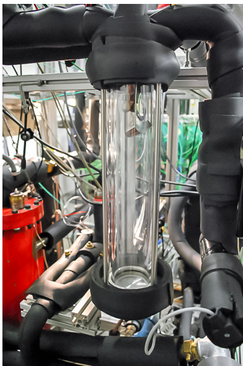
Figure B.3: First stage compressor inlet separator, in the BWP
