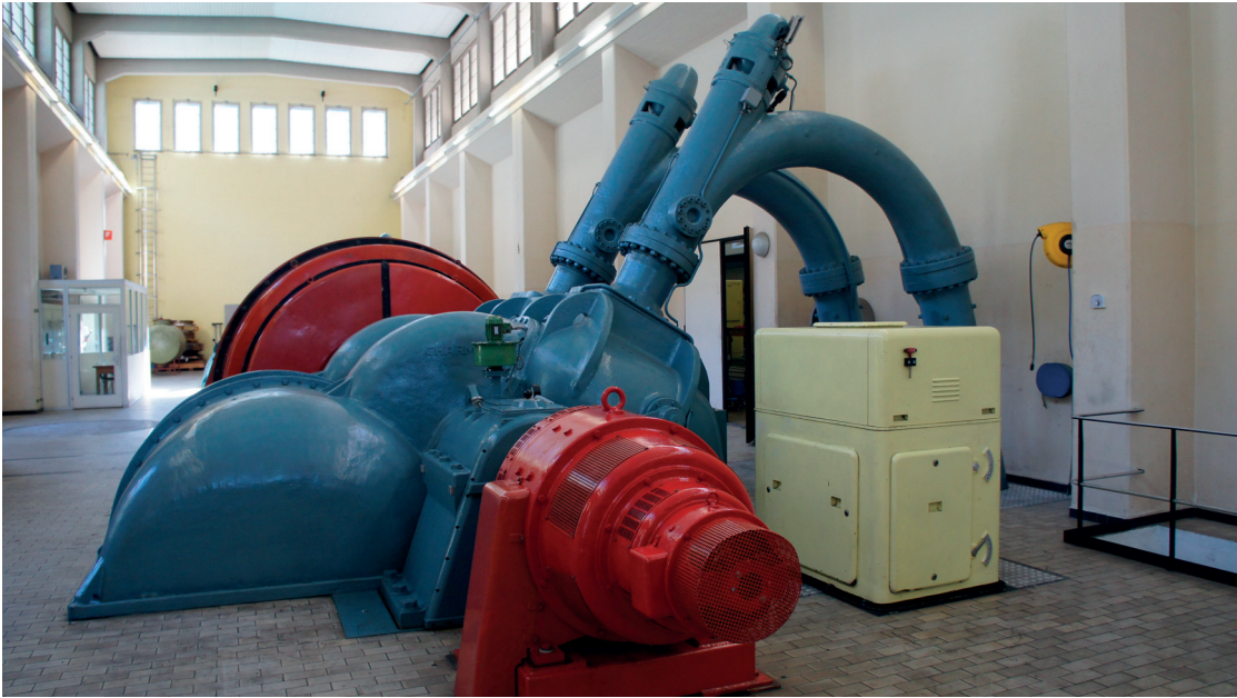
Figure 4.5: Ternary unit 3 of Mottec power plant
