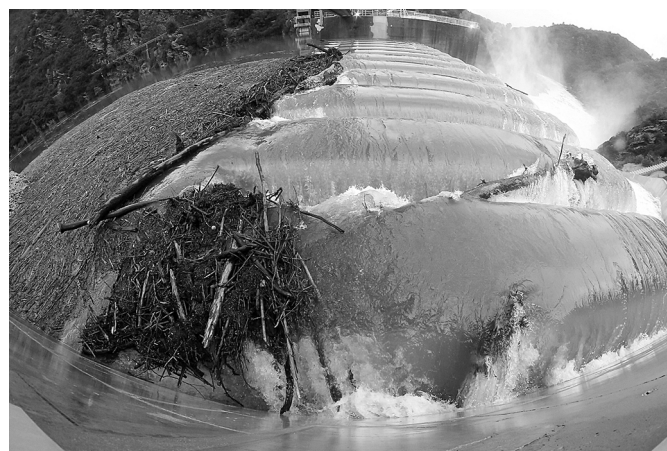
Fig. 1. Malarce Dam (F) PKW during the November 2014 flood event with debris blocking at its right part (photo: EDF France)
