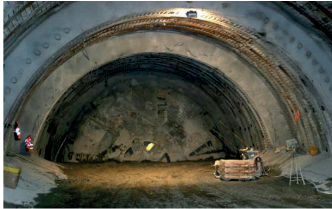
Figure 1.10 Moutier tunnel, Switzerland, the TBM cutterhead was exposed after a stop of more than two years ( http://www.a16.ch ).
