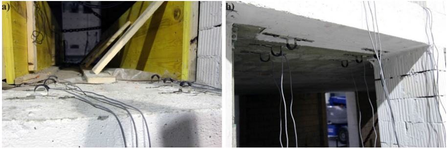
Fig. 40 Omega gages of “Location B”: top face of the slab (a) and bottom face (b)
