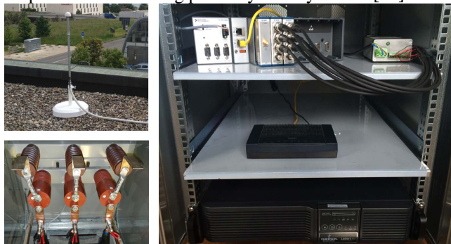
Figure 2 - EPFL-campus smart-grid components: (top left figure) GPS antenna, (bottom left figure) Altea CVS-24 current and voltage sensors and (figure on the right) rack containing the PMU (top shelf), the SHDSL modem (middle shelf) and the UPS (bottom shelf).
