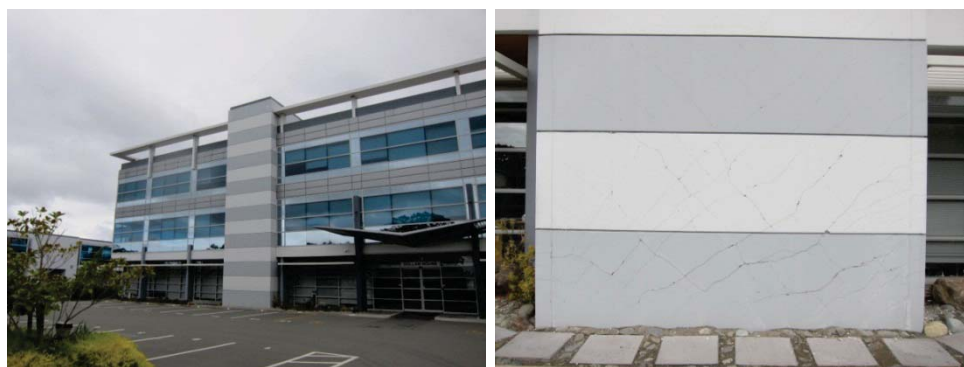
Figure 5 Observed distress to a concrete wall with minimal damage (Photos: Courtesy of Elwood)
