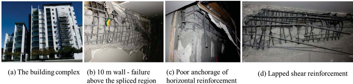
Figure 10 Performance of a concrete wall in one building of the Terrace on the Park
