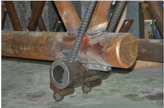
(c) Close-up of cracked joint after prestressing; crack fully closed.
