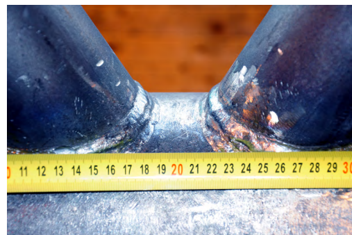
(f) Close-up of the gap at a finished joint. g^* = 23 \text{ mm}
