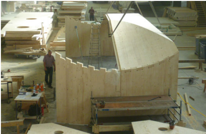
Fig. 13 Assembly of the dovetail-type connectors between the wall panels and the roof panels (Connections CV–CX)
