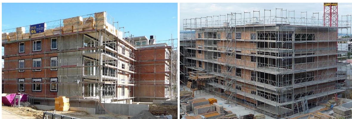
Figure 1. 3- and 6-storey residential buildings with RC wall and URM walls (Photos: Thomas Wenk).
