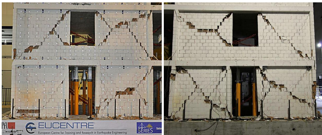
Figure 7. URM piers of the first and second storey after test number 9.
