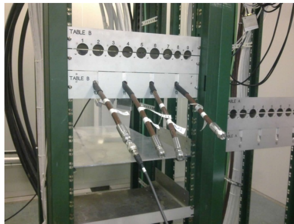
Figure 4 – The rack located in the HiRadMat control room on ground level.
