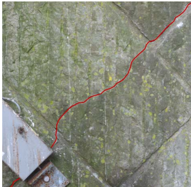
Figure 2. Emerging cracks on the arches inner side face
