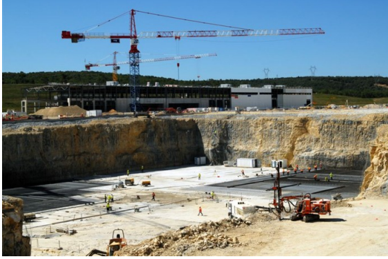
Figure 1.6: Concrete pouring for the foundation of the ITER tokamak building, 9th August 2011. Photo: F4E
