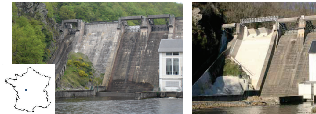
Figure 1. Downstream view of St-Marc dam with the original spillway devices (left), and with the additional PKW (right).
