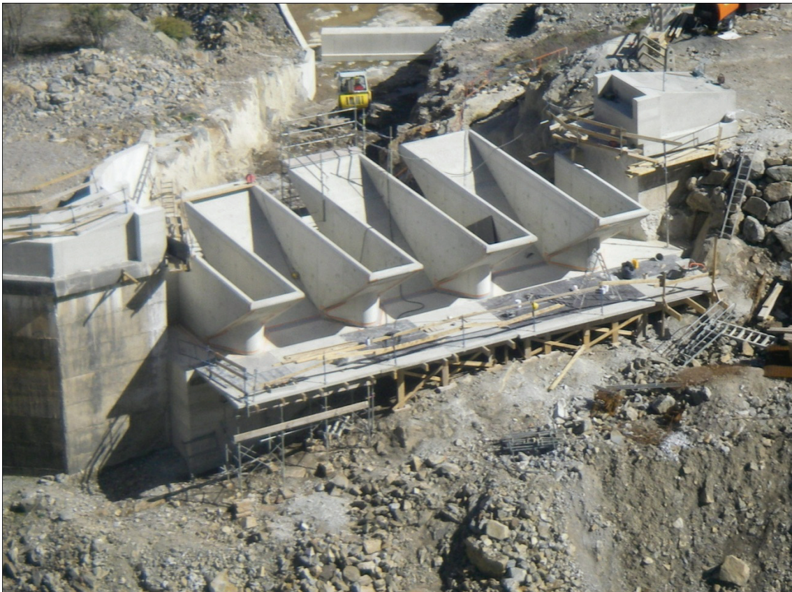
Figure 10 View of a PK weir spillway of Gloriettes dam in France during construction (Photo : EDF)
