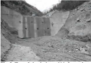
Fig 5. Toe of check dam n°11. Lateral erosion and channel deposition.
