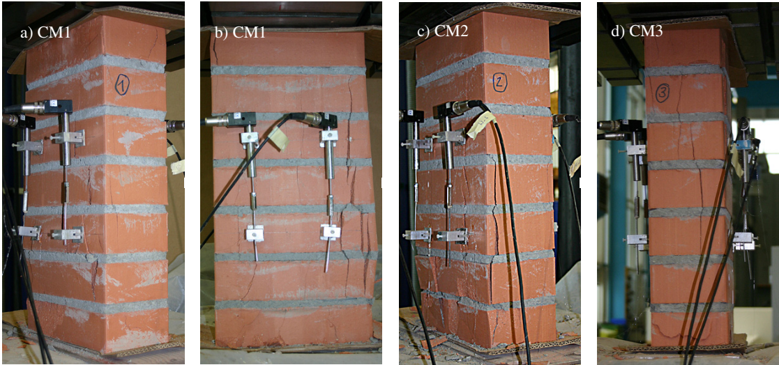
Figure 2.14: Compression tests on masonry wallettes: Crack pattern after failure for units CM1-CM3.
