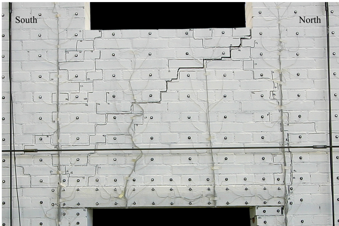
Figure 3.3: TUA: Crack pattern of spandrel at LS 23. Drift towards South with \theta_{nom} = -0.4\% .
