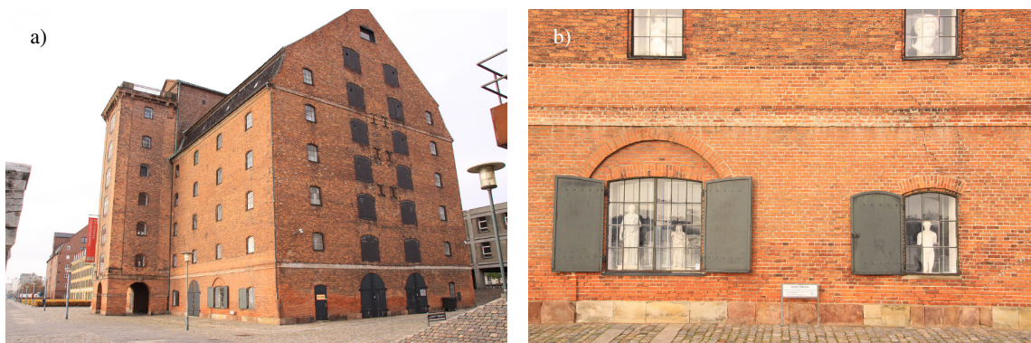
Figure 1.2: Old URM masonry house with masonry arches in the city centre of Copenhagen (Denmark): Entire building (a) and arches bridging the window openings (b).
