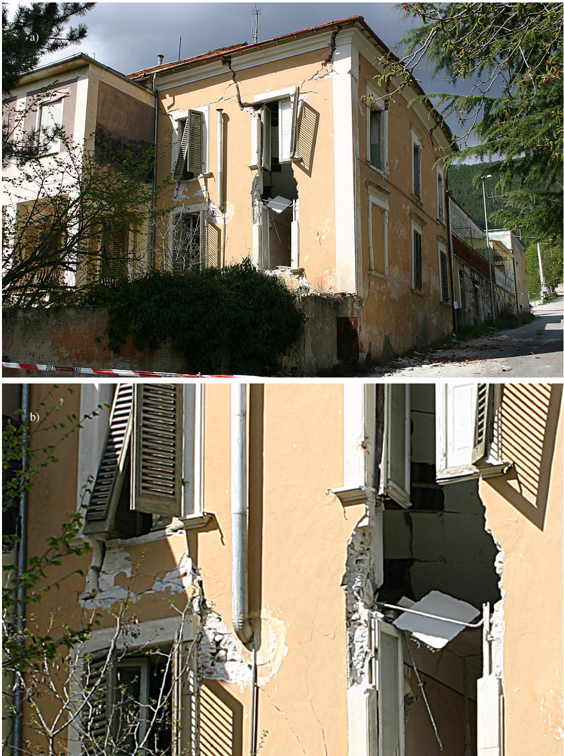
Figure 1.7: Flexural failure of spandrels in an old URM building with lintels during the L'Aquila earthquake on April 6th, 2009: Entire building (a) and detail of a spandrel (b).
