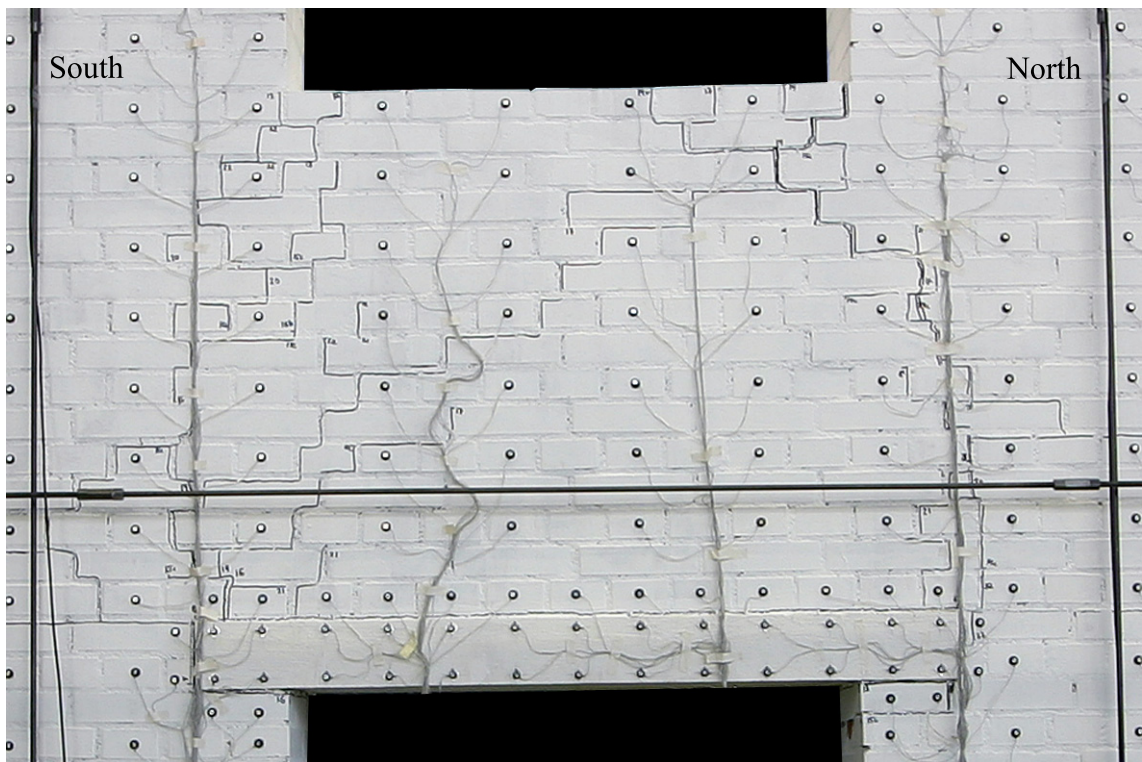
Figure 3.2: TUA: Crack pattern of spandrel at LS 22. Drift towards North with \theta_{nom} = 0.4\% .
