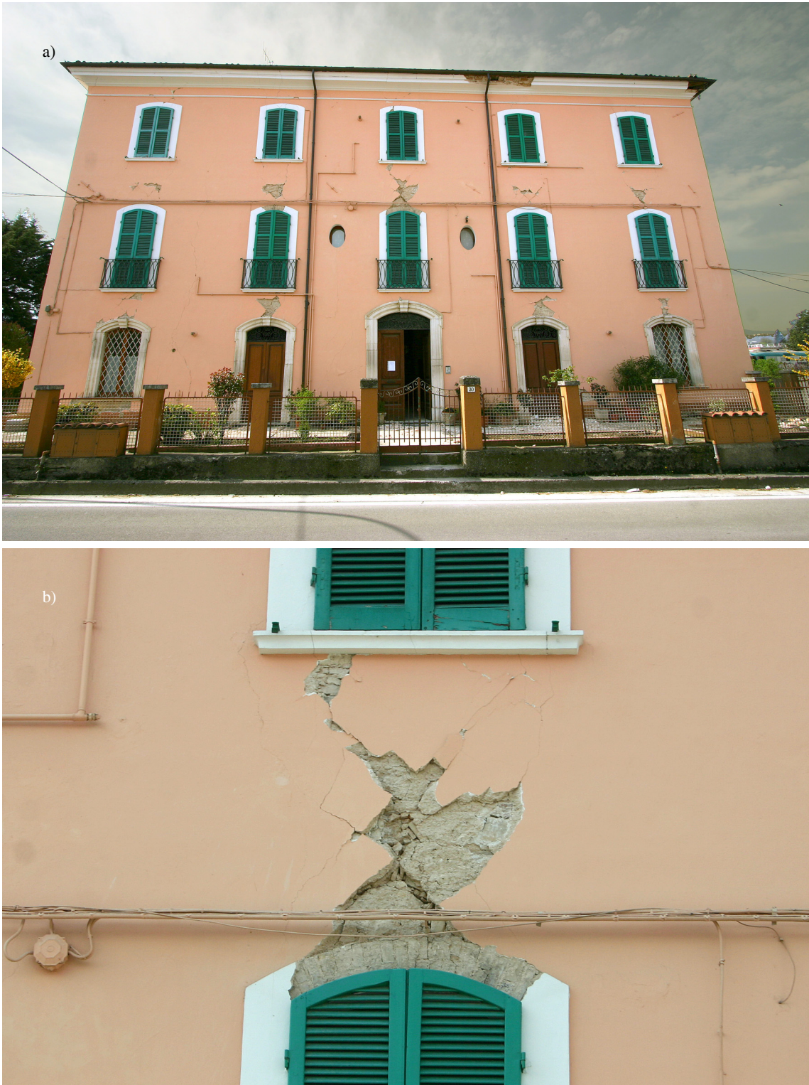
Figure 1.6: Shear failure of spandrels in an old URM building with masonry arches during the L'Aquila earthquake on April 6th, 2009: Entire building (a) and detail of a spandrel (b).
