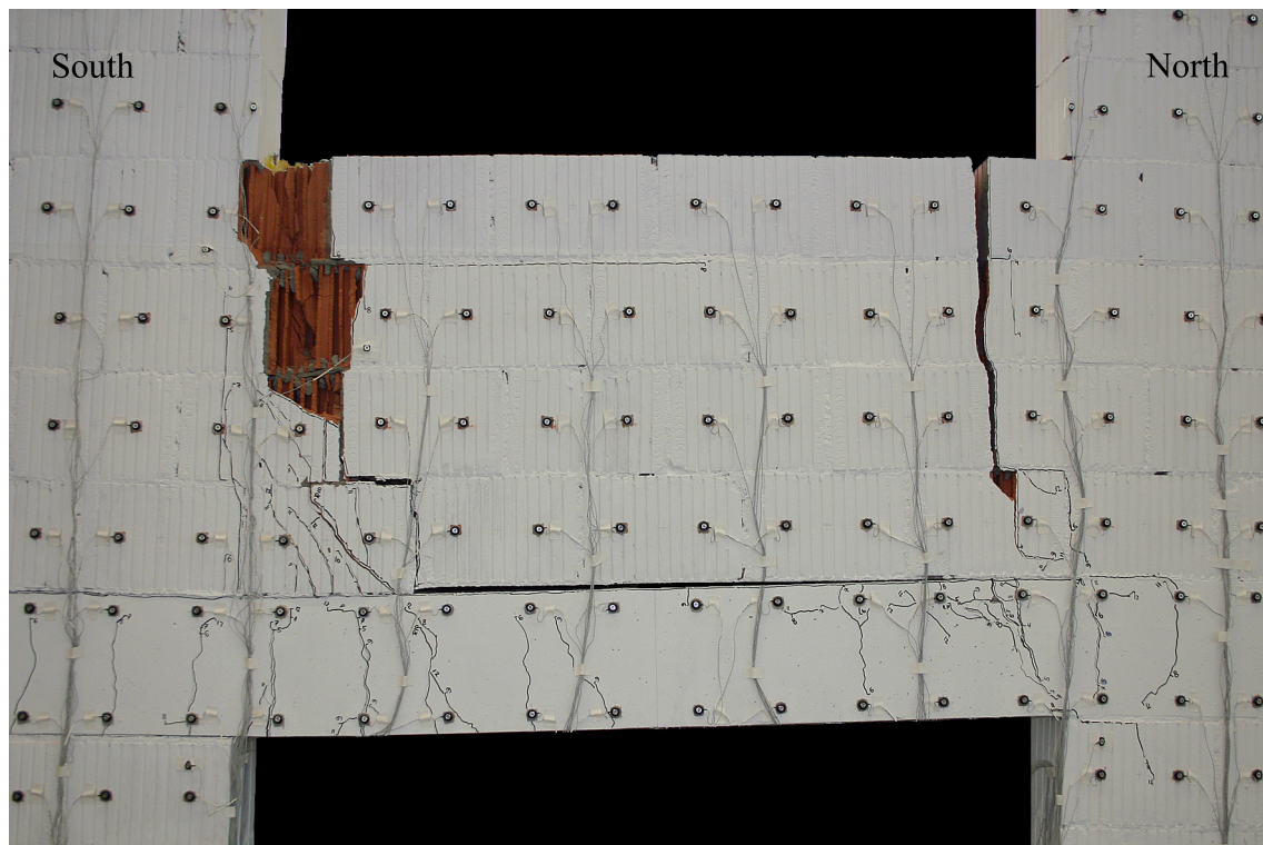
Figure 3.5: TU1: Crack pattern of spandrel at LS 12. Drift towards North with \theta_{nom} = 2\% .
