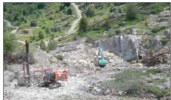
July 2009: Drilling machine, power shovel and hydraulic rock breaker during the excavation of the stilling basin.
