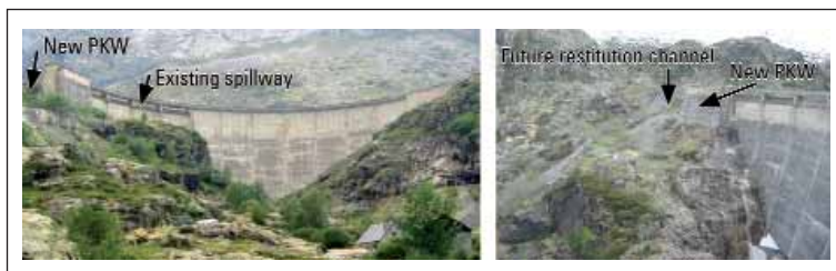
Fig. 1. Downstream views of Gloriettes dam showing the existing spillway on the left, and the right dam abutment and construction site of the new spillway on the right.
