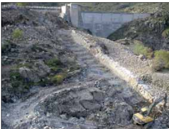
October 2009: The downstream part of the first stepped reach has been completed. The upper part of the reach (with the concrete steps) and the PKW was carried out recently.
