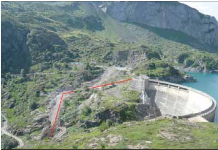
Gloriettes dam area during the excavation of the stilling basin and the channel reaches (in July 2009). The line indicates channel axis.
