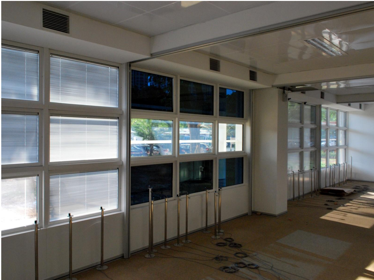
Figure 1: Facade as seen from inside with partition walls opened. From left to right: glazing integrated blinds, electrochromatic glazing, aSi photovoltaic glazing, and clear glass.
