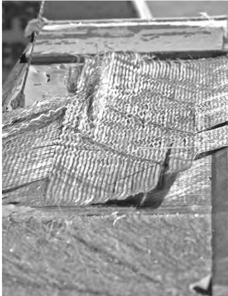
(a) Fiber mats pulled out of bridge deck surface
