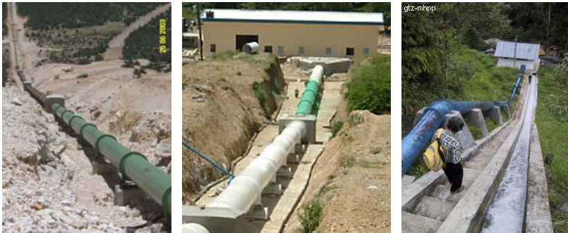
Figure 9. Examples of penstocks with supports and anchor blocks
