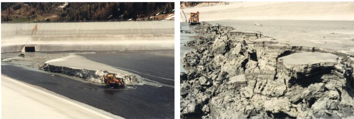
Figure 8: Dry excavation of the fine sediments (silts) in the compensation basin of Les Esserts, part of the hydroelectric scheme of Emosson
