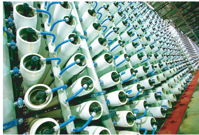
Reverse Osmosis Pressure Vessels
